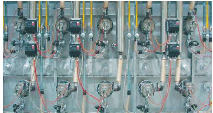
Roller hearth furnace
